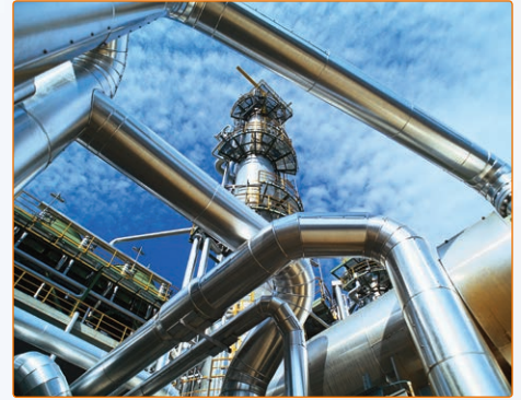
Chemical, Oil and Gas
